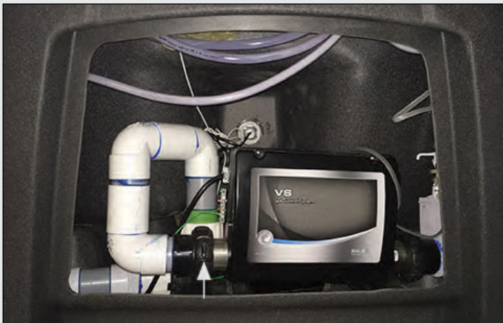
FIGURE 1.2a : HEATER UNION; LOOSEN UP TO BLEED AIR
